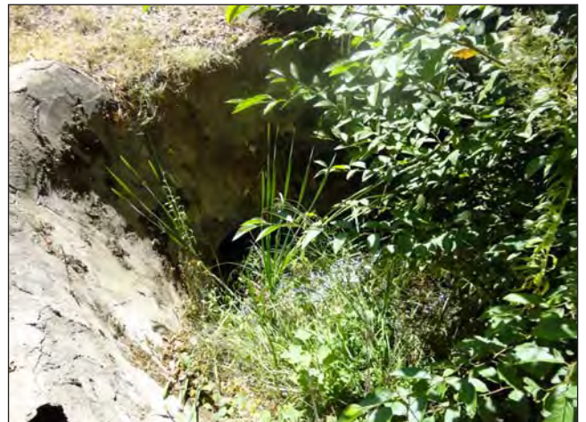
PHOTO 9: Looking at unnamed drainage on the north bank of the American River where it enters culvert.
