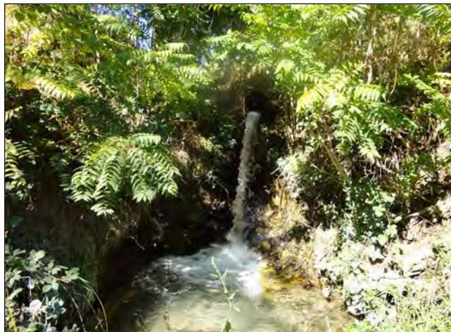
PHOTO 10: Looking at the culvert on the north bank where it drops into a plunge pool before flowing into the American River.
