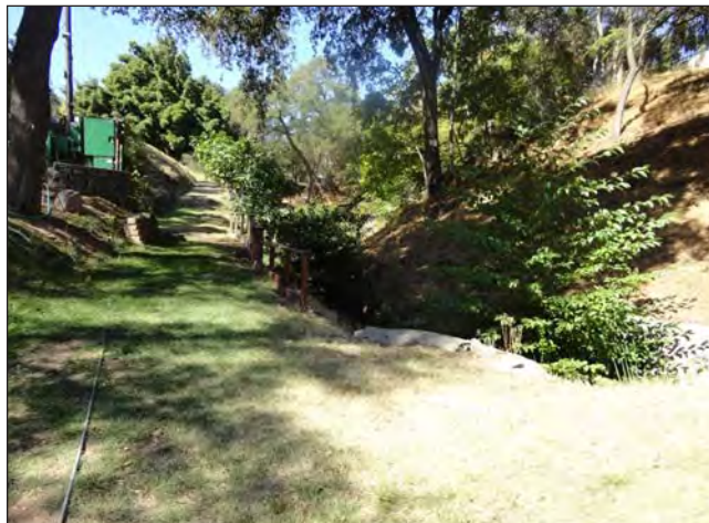
PHOTO 5: Looking north on the north bank at the intake to the culvert for the perennial drainage.
