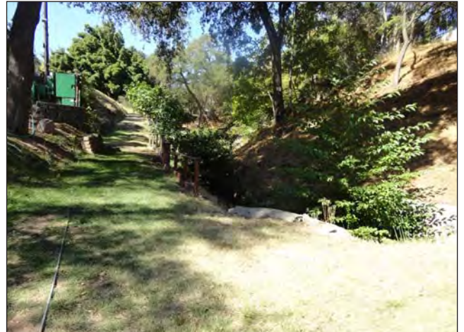
PHOTO 7: Looking north on the north bank at the intake to the culvert for the perennial drainage.
