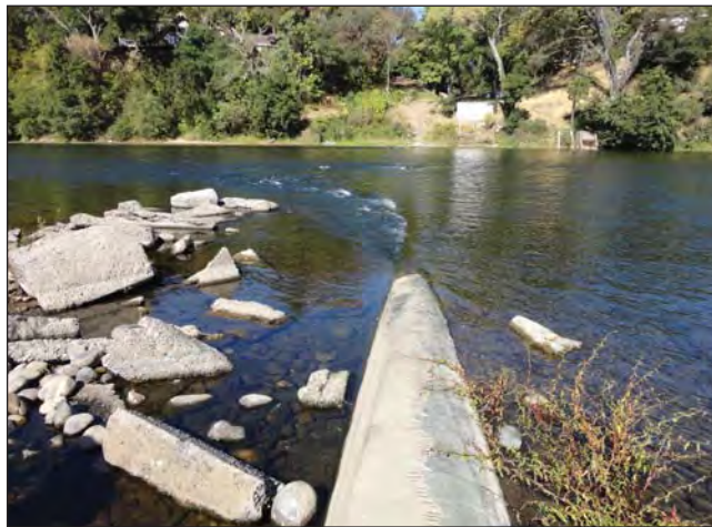
PHOTO 2: Exposed pipeline creating a safety hazard across the American River.
